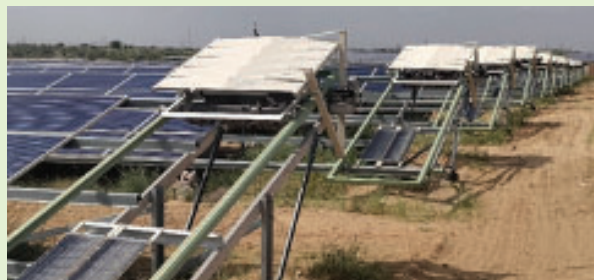
Robotic Solar Module Cleaning Technology at Bhadla
